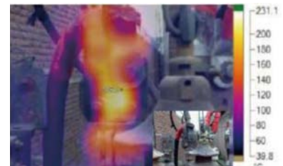
Figure 2. IR thermographic identification of a loose transformer connection. The inset is a view of the entire device.
