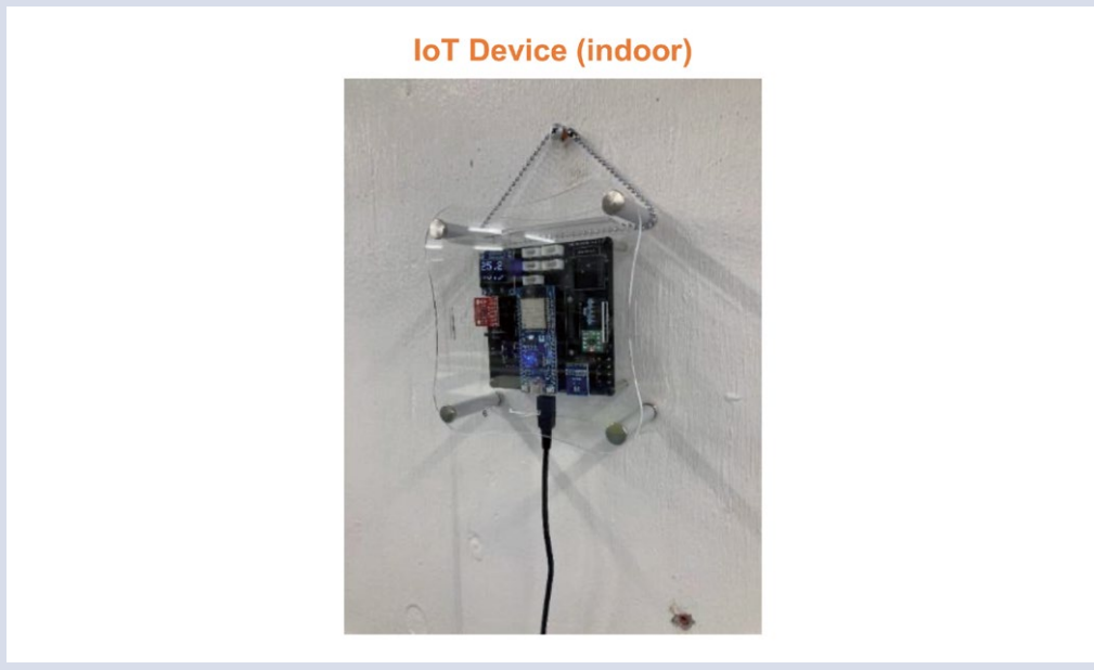
FIGURE 3-22 DEVICE INSTALLED ON THE WALL
