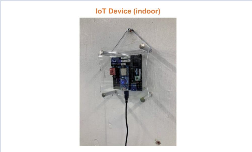
FIGURE 3-22 DEVICE INSTALLED ON THE WALL
